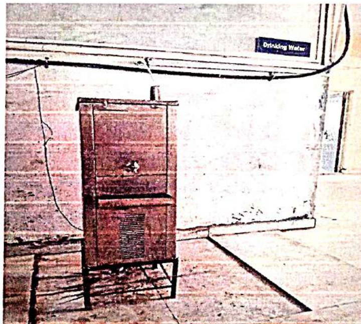
Fig. 9 Drinking Water Facility
